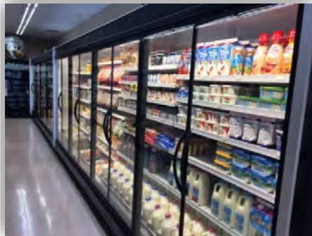
Energy Efficient Refrigeration Cases
