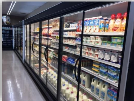
Energy Efficient Refrigeration Cases
